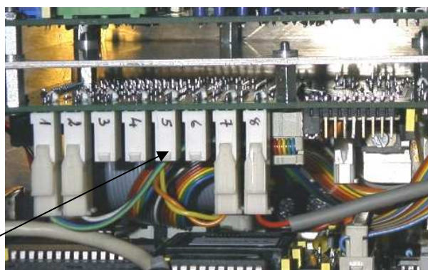
Fig 2: Control relay of the power board
