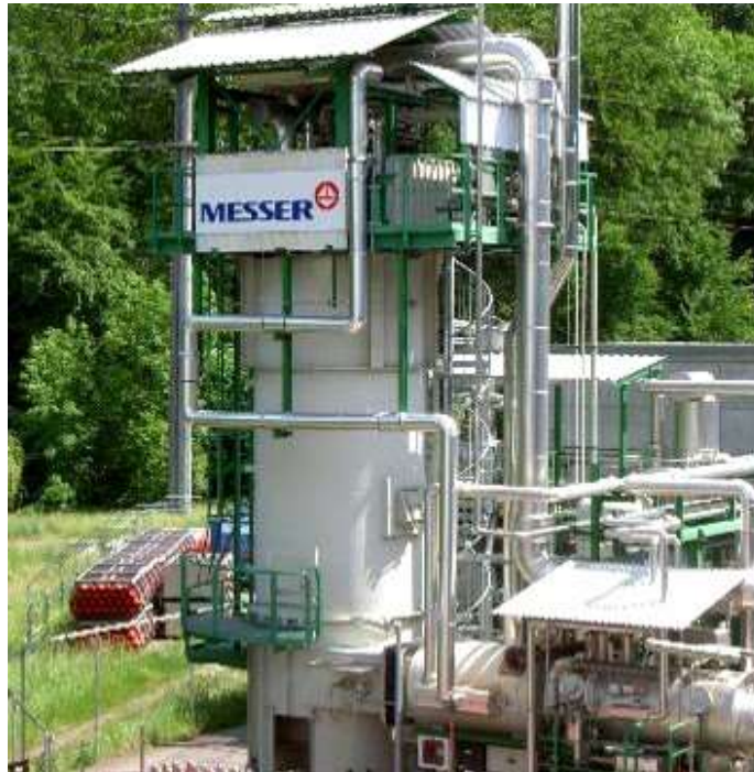
Steamreformer (Wasserstoff) Lenzburg
